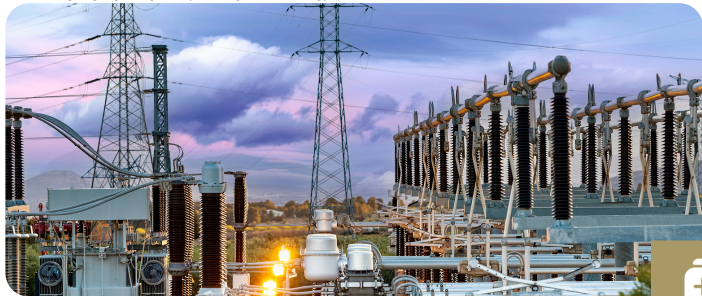
Power Distribution Plant
