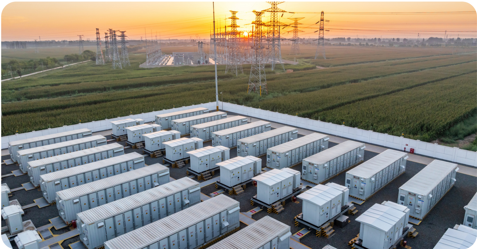
Energy Storage Power Station
